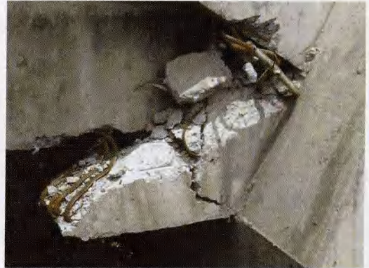
照片 8 拱肋剪切破坏 Photo 8 Shear failure of the arch rib
