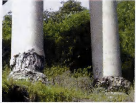
照片 2 墩底压溃 Photo 2 Axial failure of the piers
