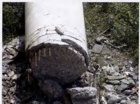
照片 6 墩底剪切破坏 Photo 6 Shear failure of the pier
