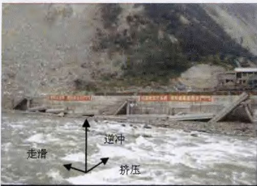
照片 5 映秀镇顺河桥 Photo 5 Collapse of Shunhe bridge in Yingxiu town
