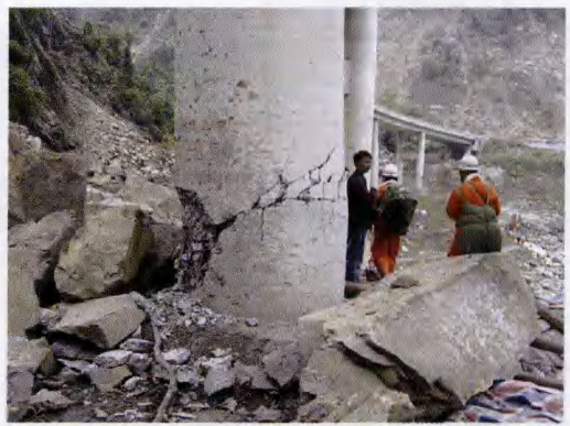
照片 4 墩底弯剪破坏 Photo 4 Moment-shear failure of the pier
