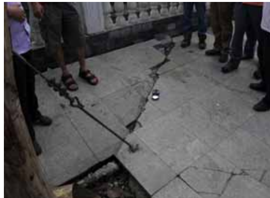
图 9 乔庄河河堤震时出现地裂缝，显示右旋走滑性质 Fig. 9 Ground fissure on the riverbank showing the dextral-slip movement near Qiaozhuang river
