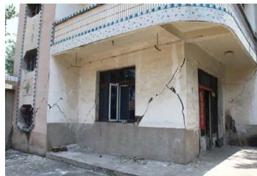
(b) 墙体“X”形裂缝
