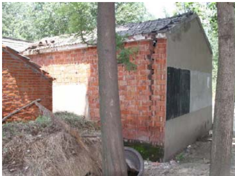
(a) 纵横墙连接处开裂
