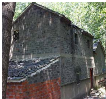
(a) 屋顶边缘瓦片被掀翻
